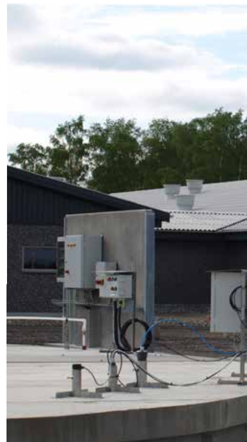
Sofiendal pig farm, machinery for manure management
